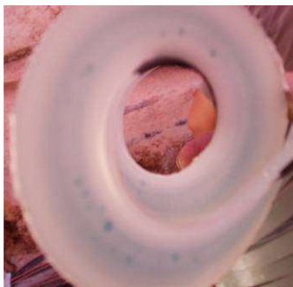
Obr. 41: Stará izolace XLPE, dutinky v kabelu XLPE, 115 kV
